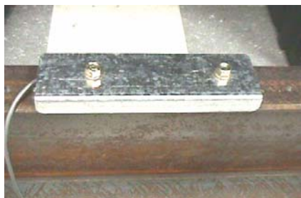
Fig 2.9 Installed sensor and cover
